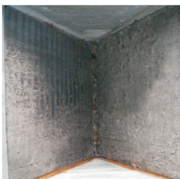
Bio-clogged HVAC cooling coil
